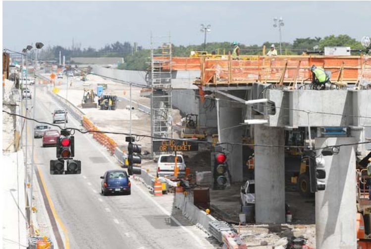
The westbound lanes of State Road 84 and the I-595 on-ramp will shift on Sunday and will run under the upper portion of the braided ramp at right while I-595 is widened. (Amy Beth Bennett, Sun Sentinel / June 27, 2011)
