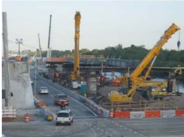
The ongoing ramp construction at the northwest corner of Pine Island Road and S.R. 84. (Source: Florida Department Of Transportation)
