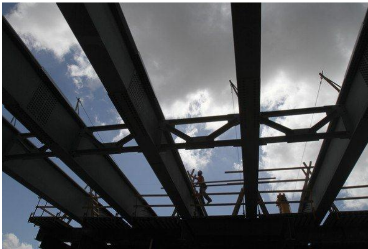
Gustavo Vargas works on the straddle pier that will support westbound I-595 lanes and the braided ramp at Pine Island Road. (Amy Beth Bennett, Sun Sentinel / April 26, 2011)
